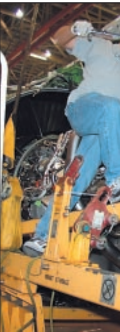
Before the platform, e 4 inch beam six feet u each bolt. Note how th
