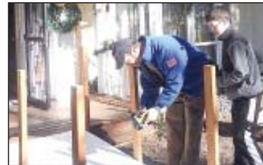
Glen Howard and his son Caleb were two of the volunteers working on the ramp project.
