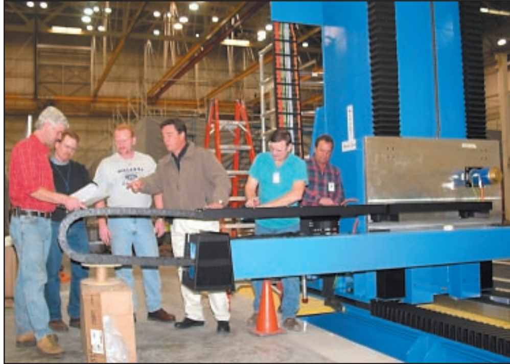
Facilities members at DC are installing an Automated Ultrasonic Scanning System to use on composites, which will cover 7800 square foot work area. No subcontractors are on site working on the installation. L to R: Dale Crueger, Marty Shepard, Chuck Fromong, Business Rep Stan Johnson, Terry Leonard, and Lynn Weaver.
