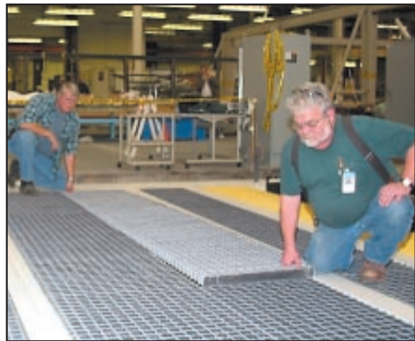
Mark Whitley (l) and Steve Chilcott were two millwrights that built the grates and did much of the concrete work on the job.
