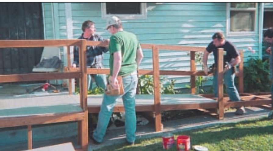
...s constructed a wheelchair ramp in November for a resident living in the Hill area. A neighbor also had a need and saw the ramp so volunteers and built the second ramp in December.
