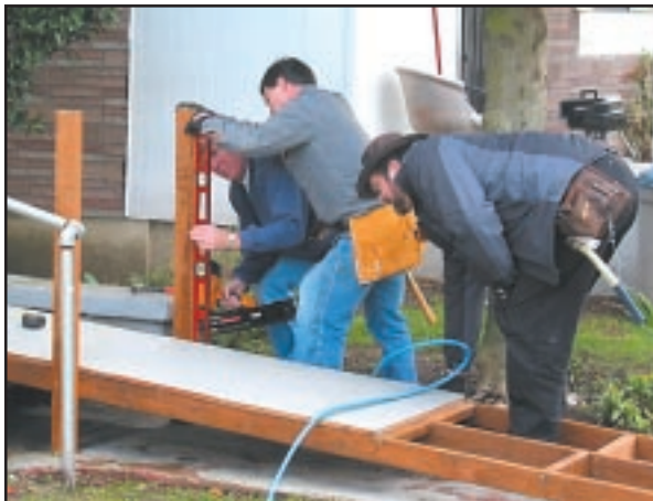
In December, members built a ramp for a second Beacon Hill resident.
