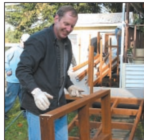
Darrell Andrews works on the frame for a recent wheelchair ramp project.
